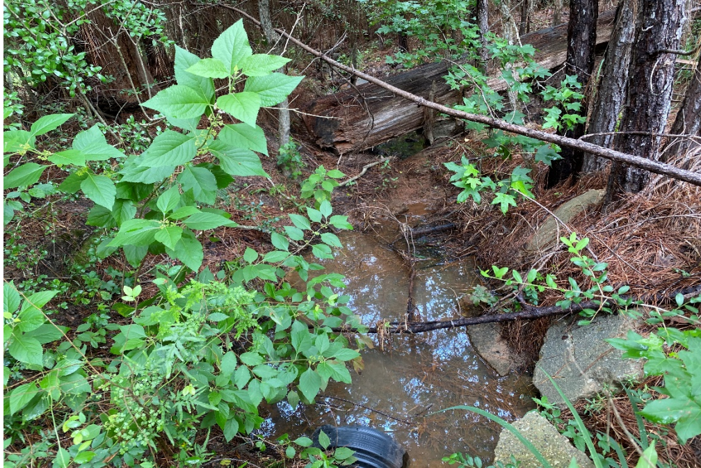
Photo 05 Photo of culvert connected to south neighboring sediment pond located on west side of subject site.
